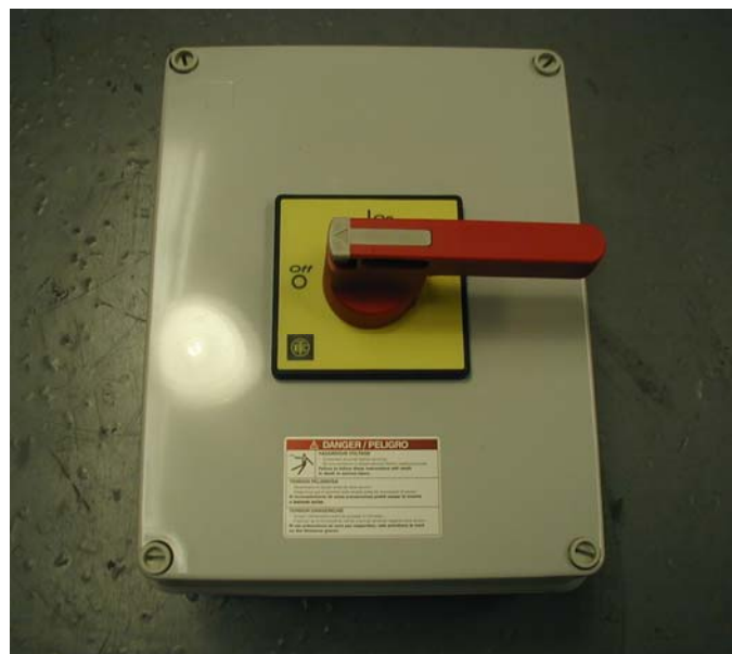
Figure 3.05-06, Main Power Disconnect Switch
