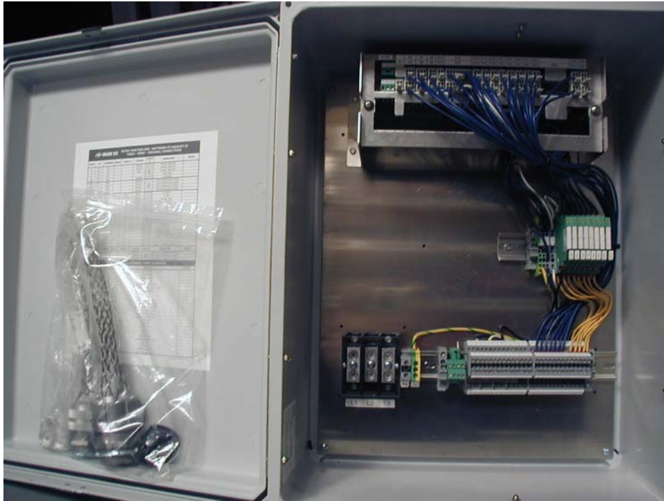
Figure 3.05-05, In-bay Junction Box
