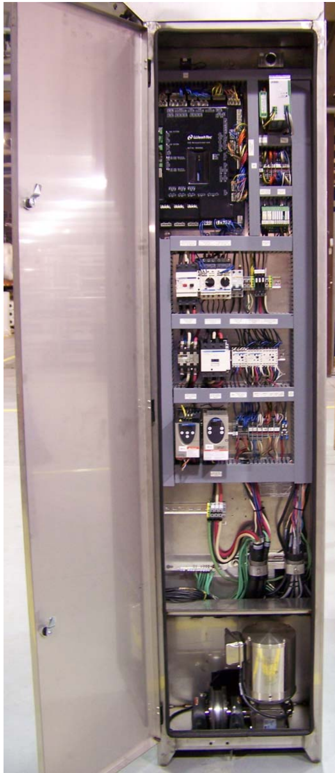
Figure 3.05-02, Main Electrical Enclosure
